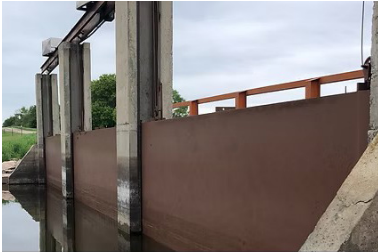
Figure B-6: Lake Poinsett Outlet Gates
