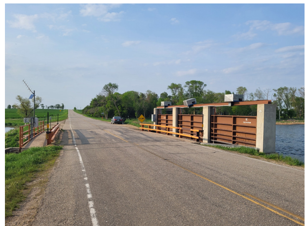
Figure B-4: Lake Poinsett Outlet Gates
